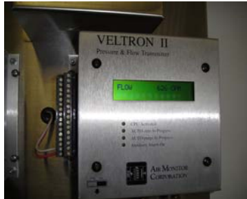
Test Room Airflow Control
